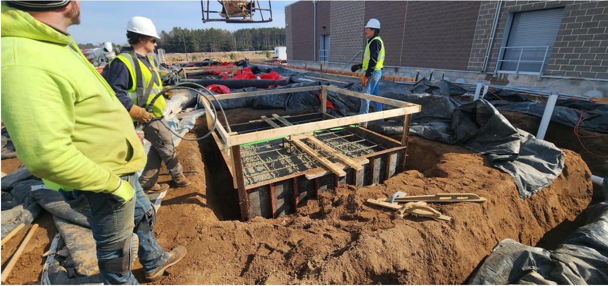
Rebar set and concrete pours concluded for the three center column support foundations in Structure 120.
