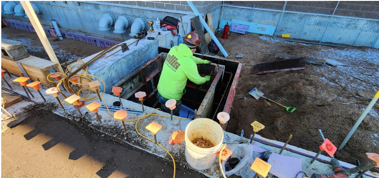
South side door stoop foundation walls for Structure 120 rebar set and formwork installed.
