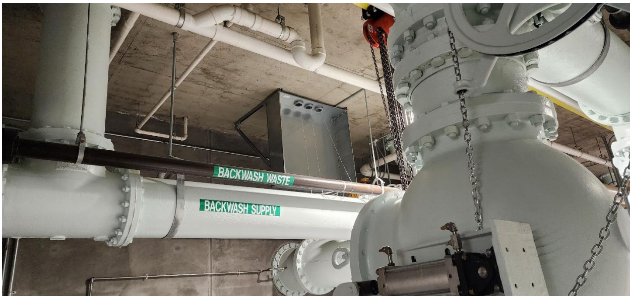
Three 4" electrical conduit runs cored through floor and junction box set to bring power to the three new Filtered Water Pumps in the basement of Structure 100.
