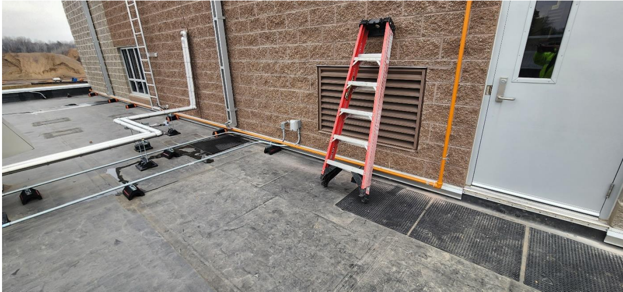
New 1" Natural Gas line installed on roof of Str 100 to provide gas to Structure 120.
