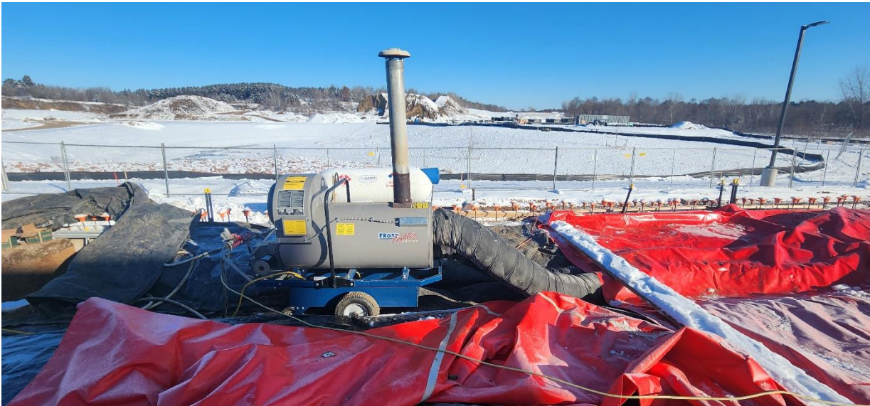
Indirect heat has been utilized to ensure rebar, structural fill and any concrete stays warm and above 32°F.
