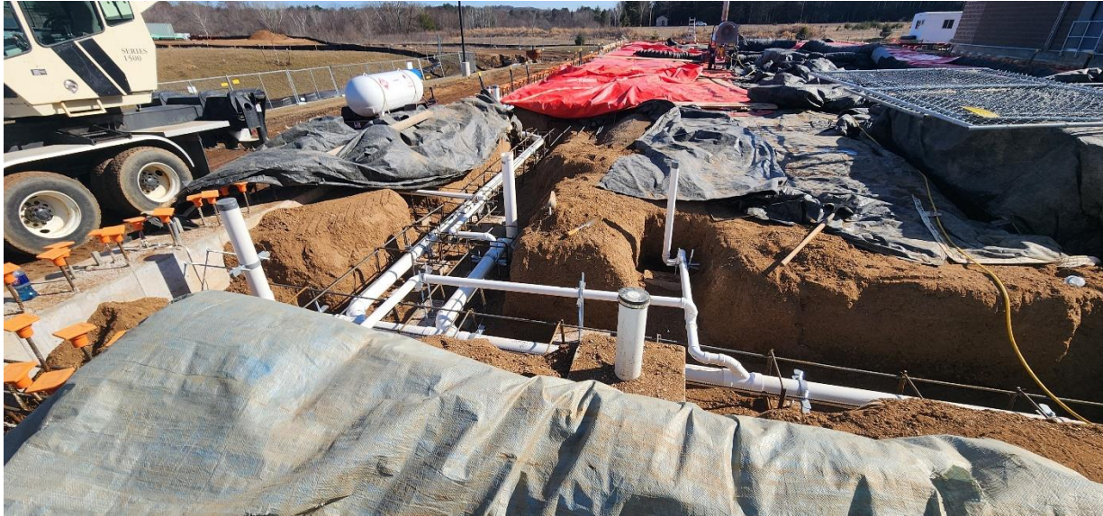
Underslab sanitary and venting installed in Structure 120, rebar formwork started for concrete encasement.
