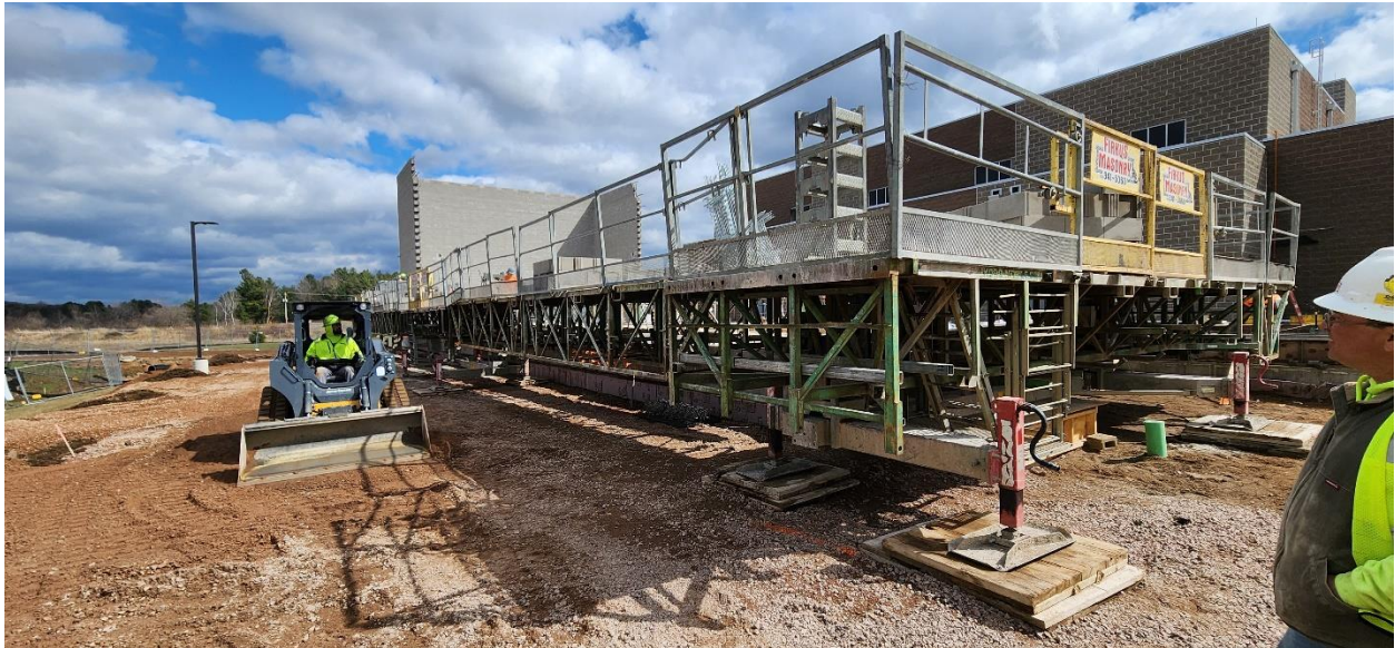
Firkus Masonry setup on the north side to continue concrete masonry unit walls for Structure 120 (PFAS Treatment Building).
