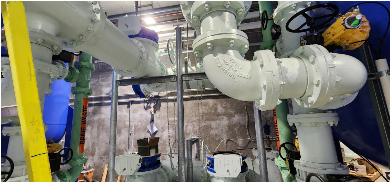
August Winters set the first pipe stands in Structure 100 (Process Building) for connection to PFAS treatment system in Structure 120.
