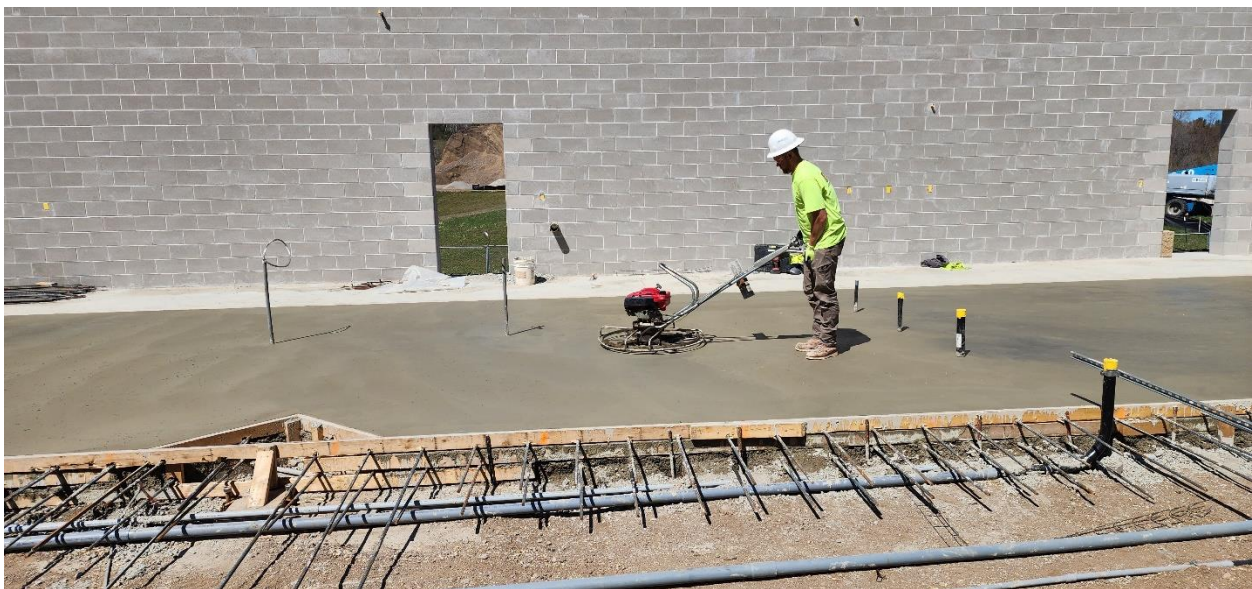
Finish work on the north portion of slab on grade in Structure 120.
