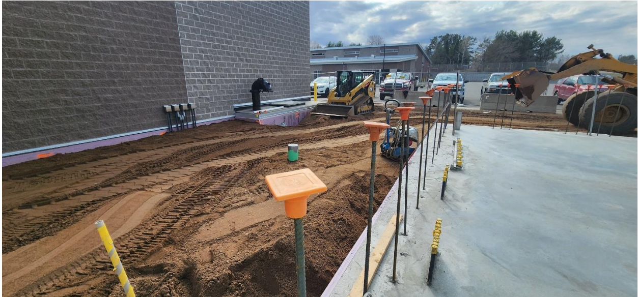
Raising the grade between Structure 100 and Structure 120 at the west side to allow for masons to set up scaffolding.
