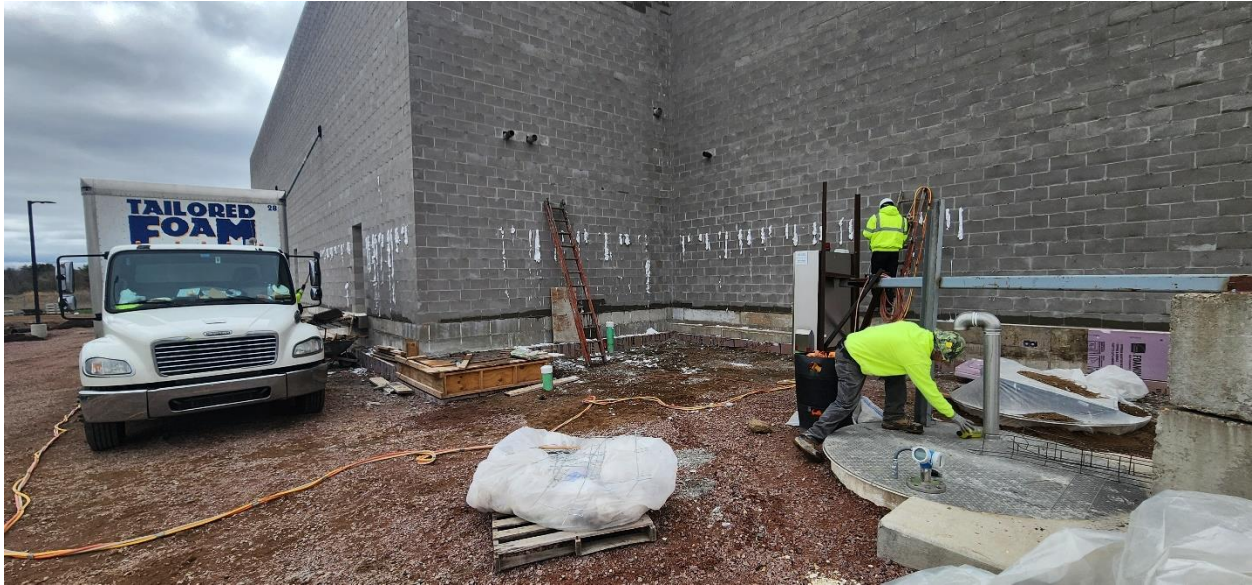
Tailored Foam injecting CMU with foam insulation at the NW corner of Structure 120
