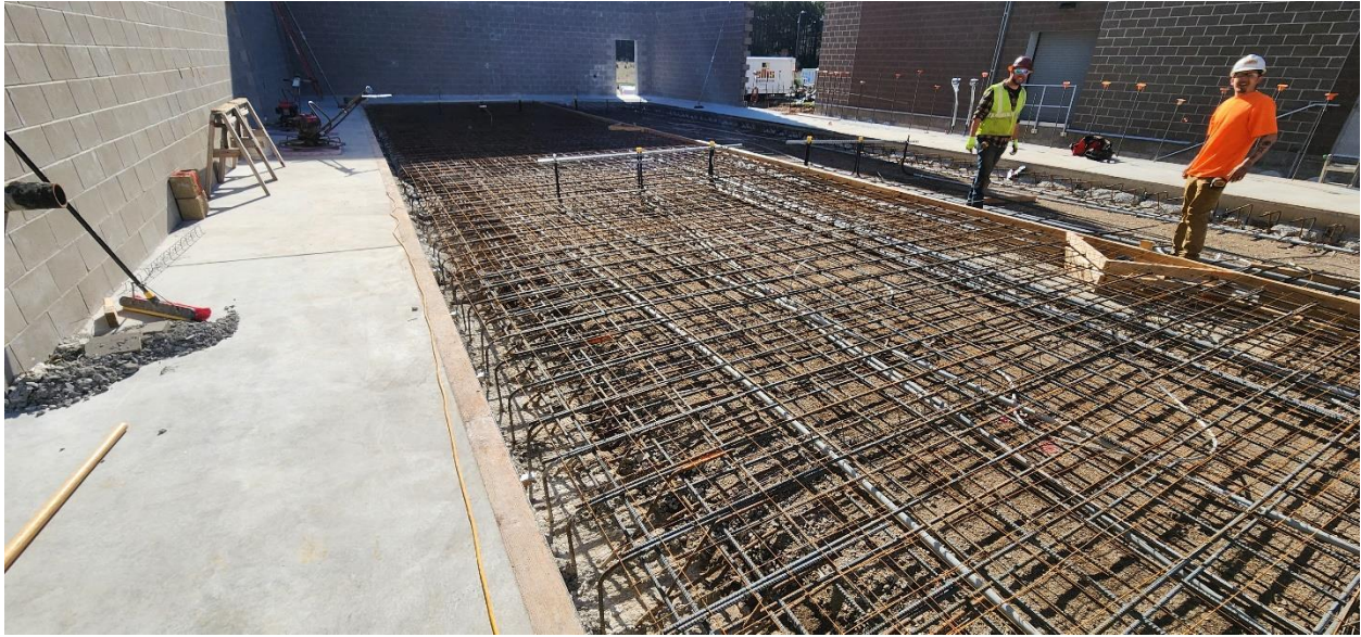
Ellis working on the rebar placement for the center north half of the slab on grade in Structure 120.
