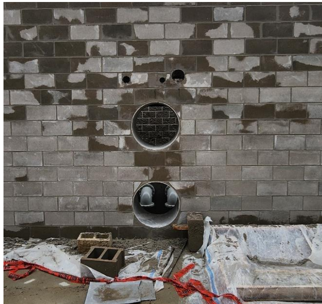
Pipe sleeves set for the two 20-inch pipes, the 4-inch W2, 1-inch natural gas and 3/4-inch W1 lines in Structure 120.
