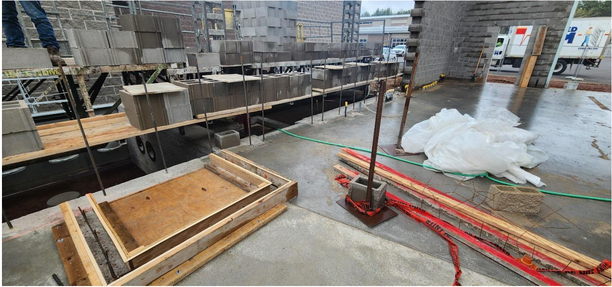
Firkus Masonry setting up to complete the south concrete masonry unit portion of the wall of Structure 120, Ellis has sump curb wall formed.
