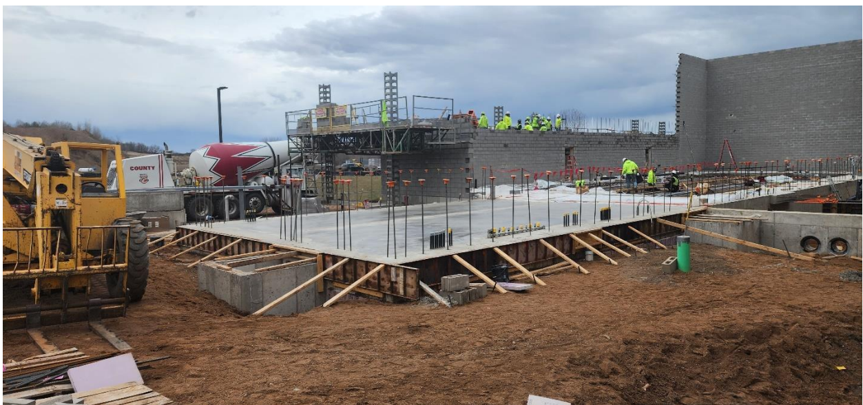
Firkus Masonry pouring first bond beam at 10-ft for the north wall of Structure 120.
