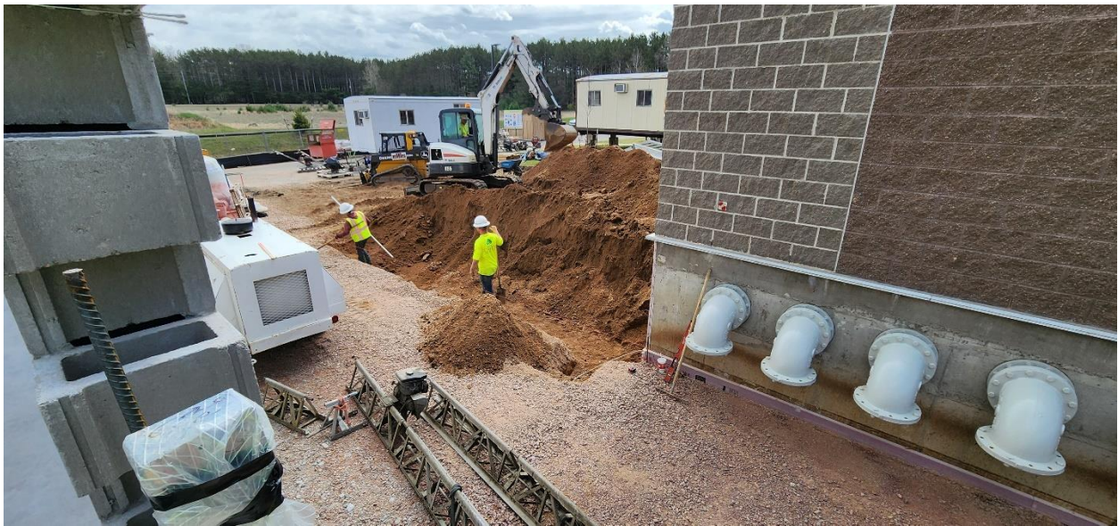
Carl's Landscape preparing the grade for the landscape retaining wall off the northeast corner of Structure 100.
