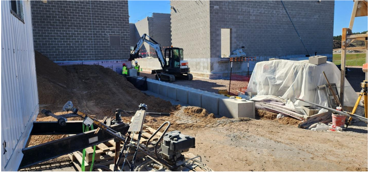
Carl's placing the concrete landscape blocks at the northeast corner of Structure 100.
