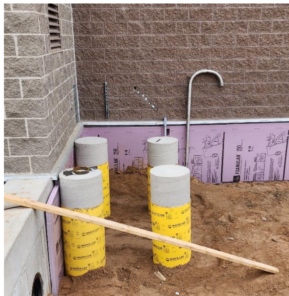
Upper pipe stand sonotubes poured between Structure 100 and Structure 120, vent pipe goose neck installed.
