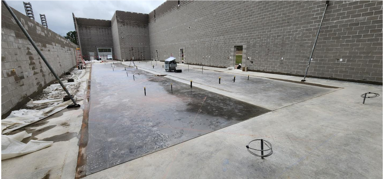
Looking west inside Structure 120 completed slab on grade, August Winter getting prepped to layout stands and piping.
