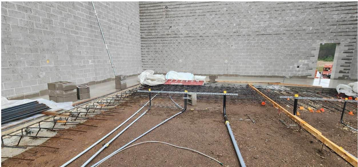
Econ Electric setting electrical conduit runs that come up through floor in Structure 120.
