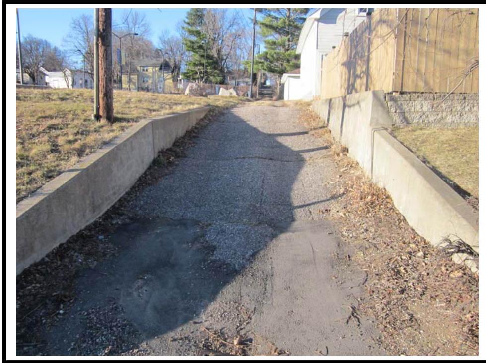
7. Neighborhood view facing north along the alley that adjoins the east side of the subject.
