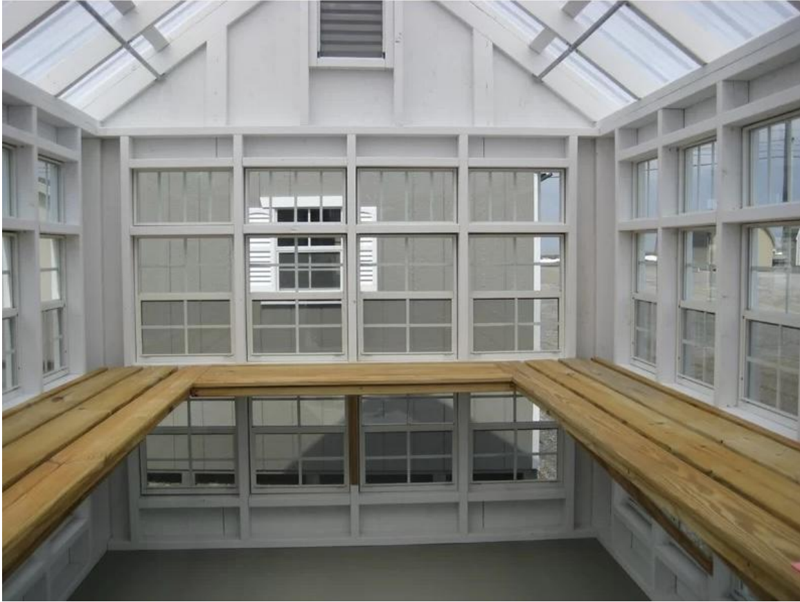
(H) A greenhouse addition will create additional communal space as well as a growing space.
