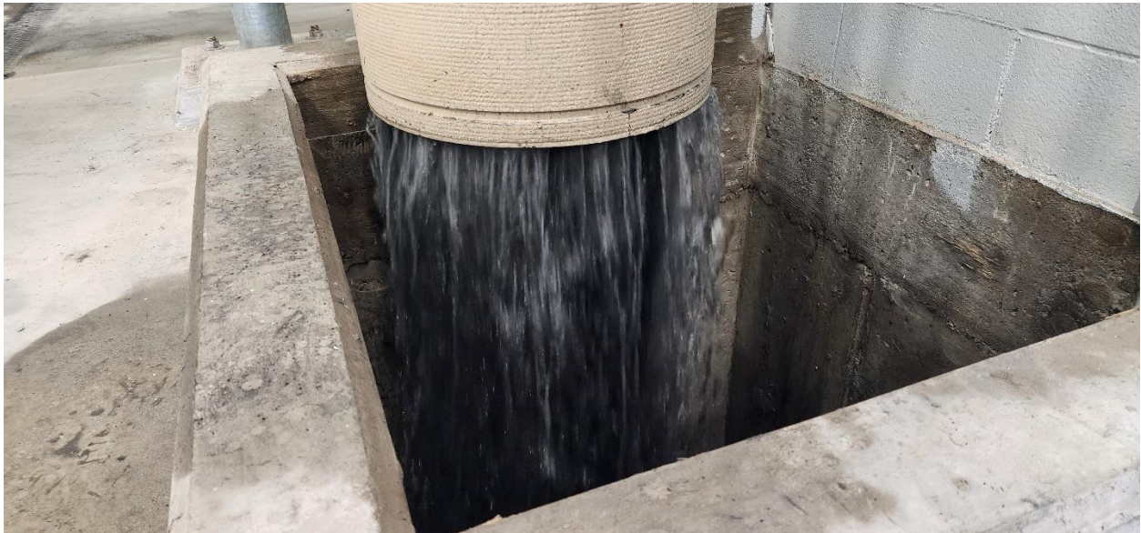
Backwashing of GAC in vessels has started, this is the GAC fines being washed out into the Structure 120 (PFAS Treatment Building) process waste sump.
