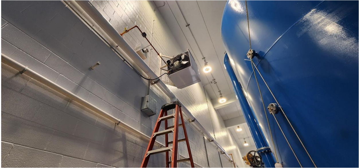
Structure 120 (PFAS Treatment Building) gas unit heaters installed and prepping for wiring power and control to each unit.
