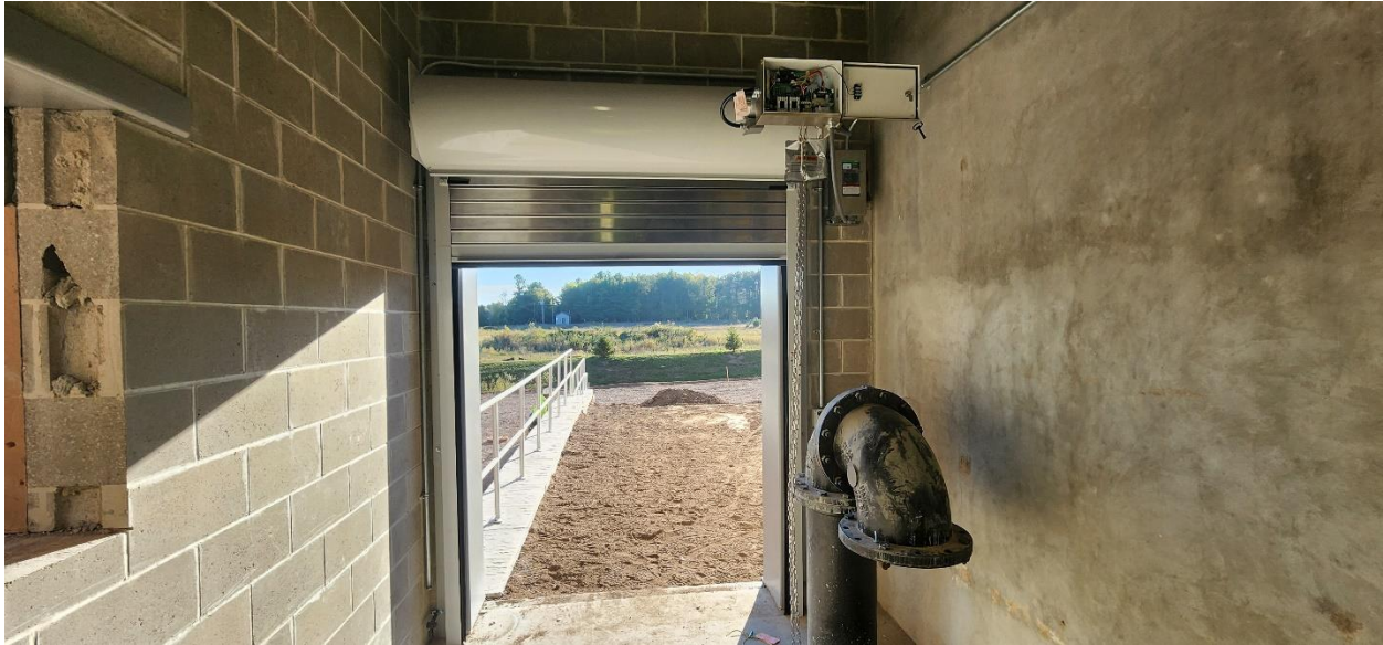
Structure 100 (Process Building) new overhead garage door installed in storage area located north of the Filtered Water tanks.
