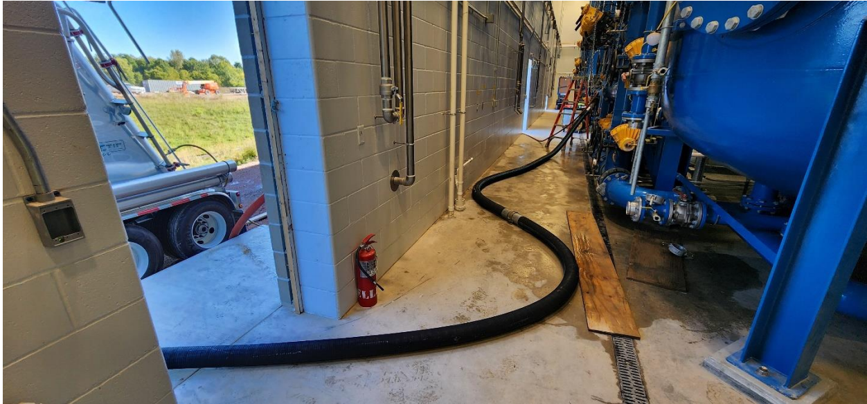
Structure 120 (PFAS Treatment Building) 46,000 lbs. of granular activated carbon (GAC) being installed into one PFAS vessel by Calgon (11 more to go).
