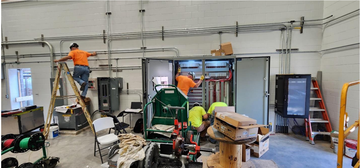
Structure 120 (PFAS Treatment Building) network rack and 120-PLC installed and wired.
