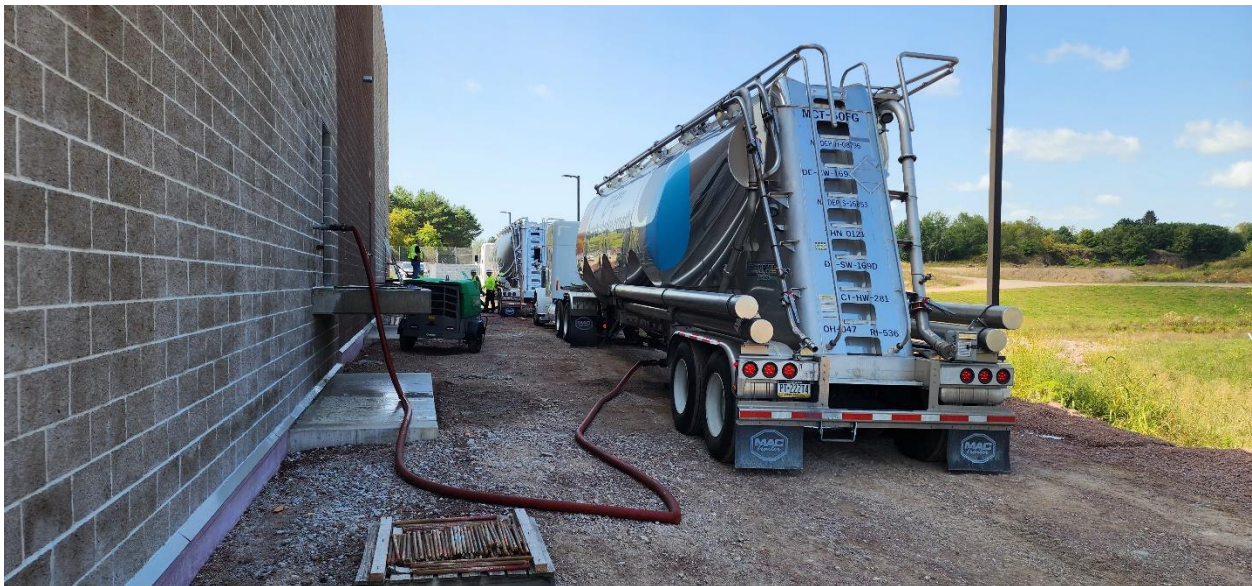
Pumping water into GAC tanker truck to suspend in order to pump into GAC vessels.
