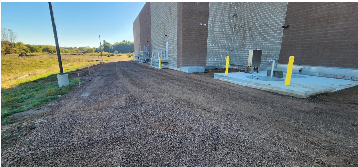
Structure 120 (PFAS Treatment Building) man doors and stairways installed, rough grade for asphalt completed, and concrete poured for Structure 410 slab, Structure 120 (PFAS Treatment Building) exterior sump and for landings below man doors.
