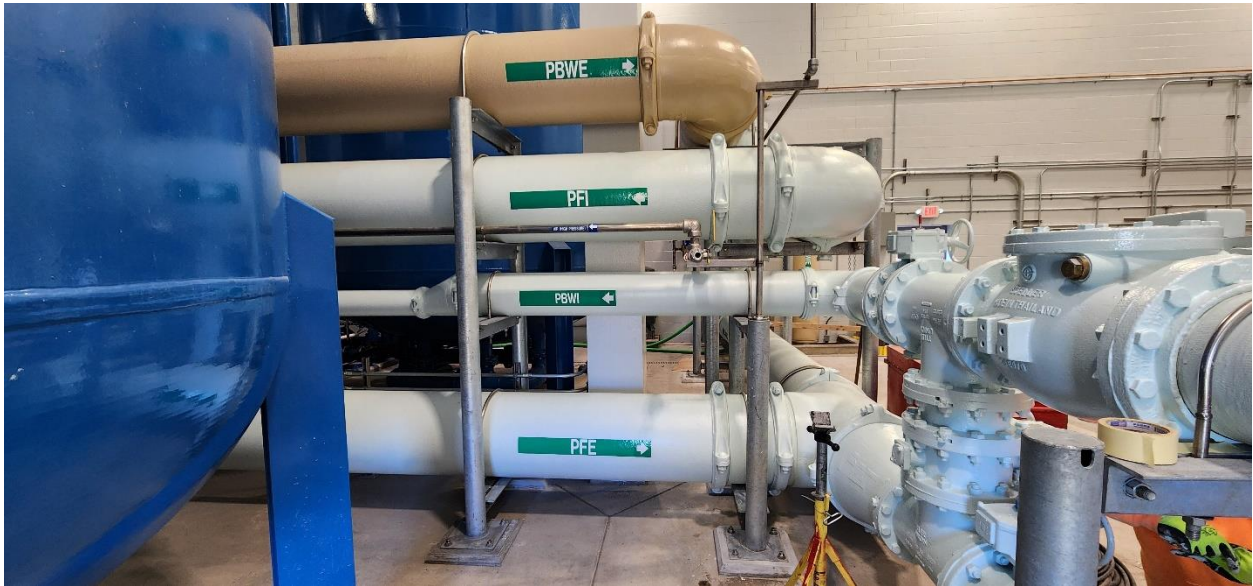
Structure 120 (PFAS Treatment Building) Pipe labelling ongoing.
