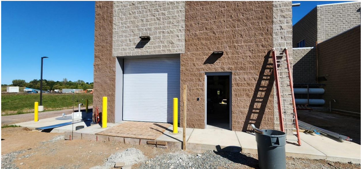
Structure 120 (PFAS Treatment Building) overhead garage door, building pipe bollards and exterior lighting installed.
