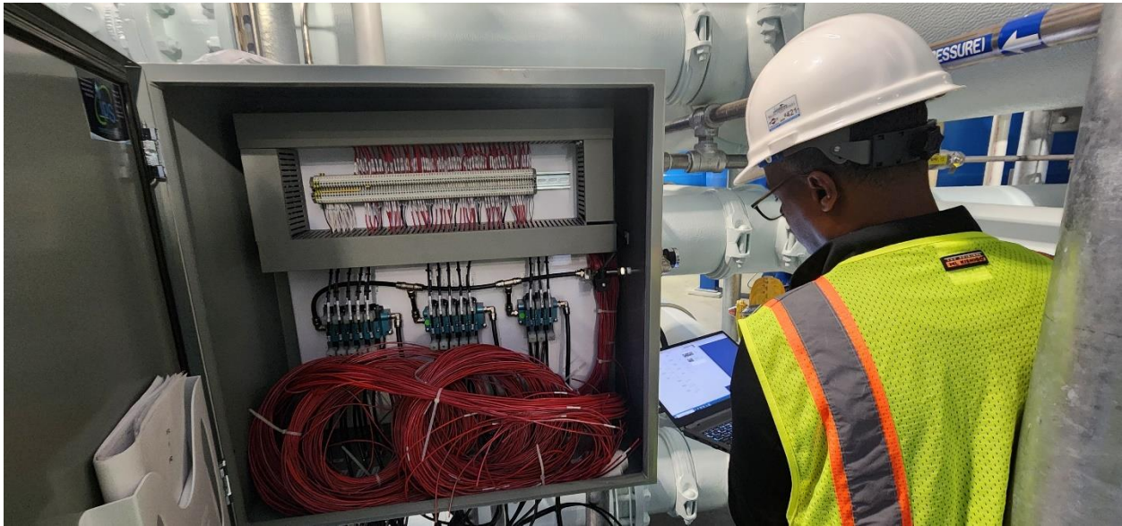
Structure 120 (PFAS Treatment Building) Donohue SCADA Programmer working with Aqueous Vets and IPS to set up the actuated valves on GAC vessels.
