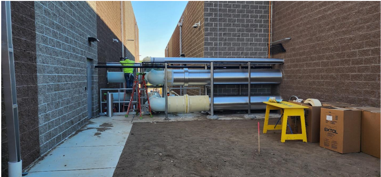
Exterior piping between Structure 100 (Process Building) and Structure 120 (PFAS Treatment Building) getting pipe insulation and jacketing installed.
