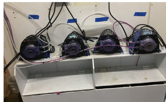
Chemical Metering Pumps
