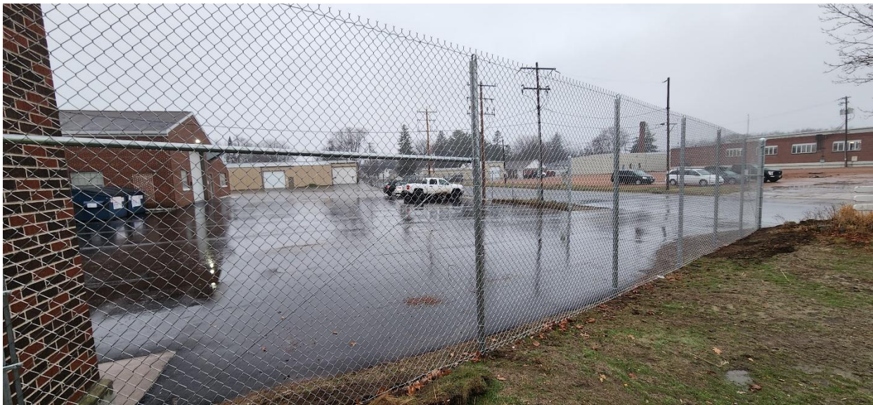
Final fence work from Structure 100 (Main Building) to Adrian Street; waiting on new gate.
