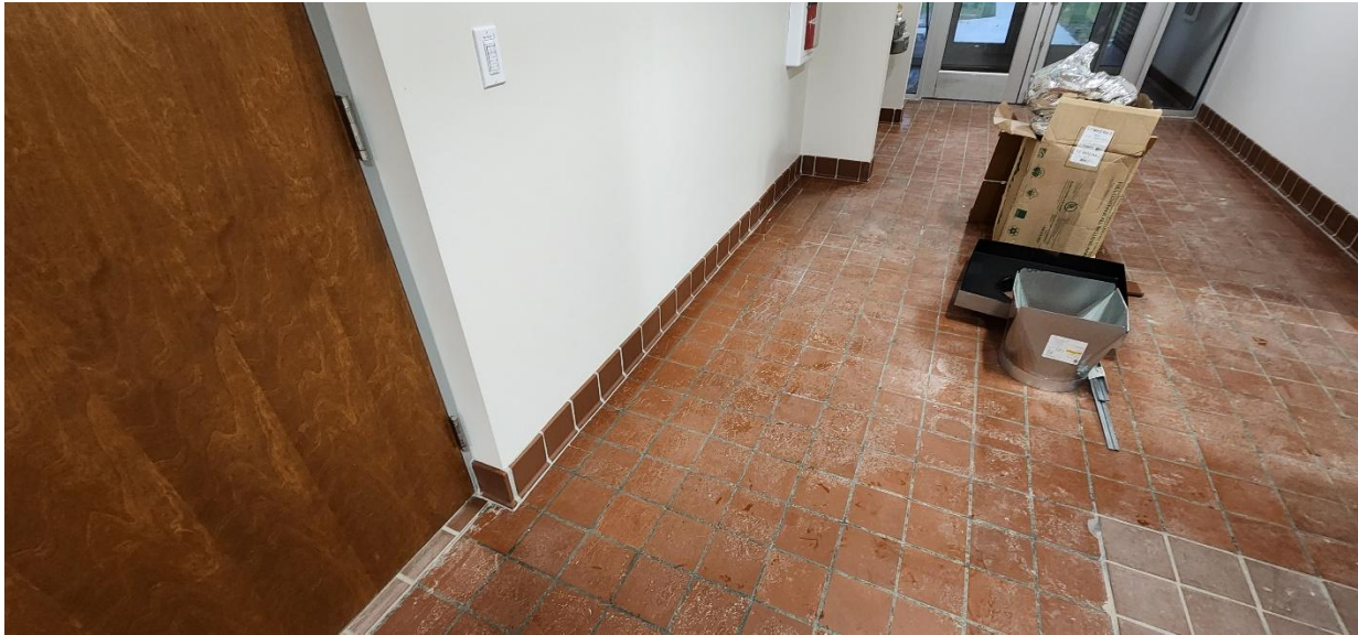
Tile baseboard work completed in foyer area and hallway of Structure 100 (Main Building).
