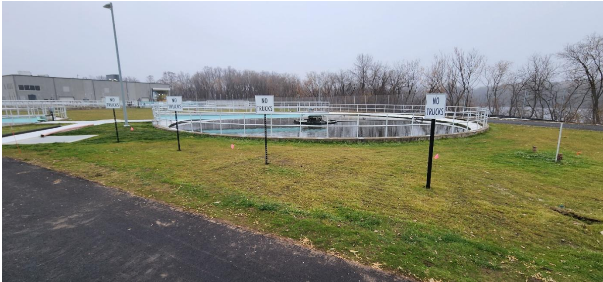
“No Truck” signs placed at Structure 520 (Secondary Clarifier 2) for shallow buried 48-inch secondary effluent line.
