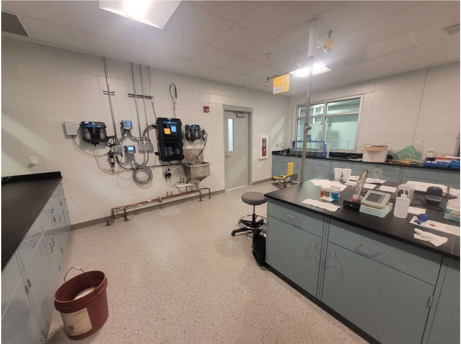
Drinking Water Treatment Facility Lab Analyzers and Equipment
