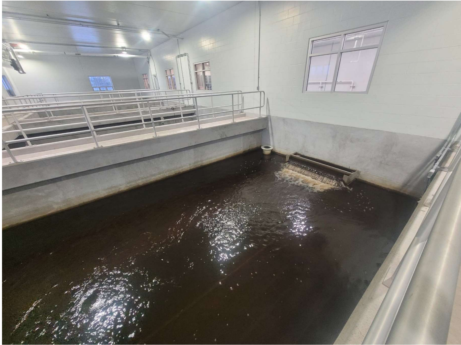
Influent Water to Top of Greensand Filters Post Aeration and Clarification
