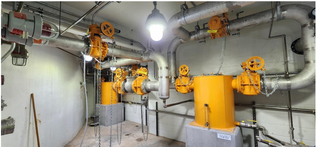
Newly painted valves and condensate tanks in gas handling room of Structure 700 (Digester Building).
