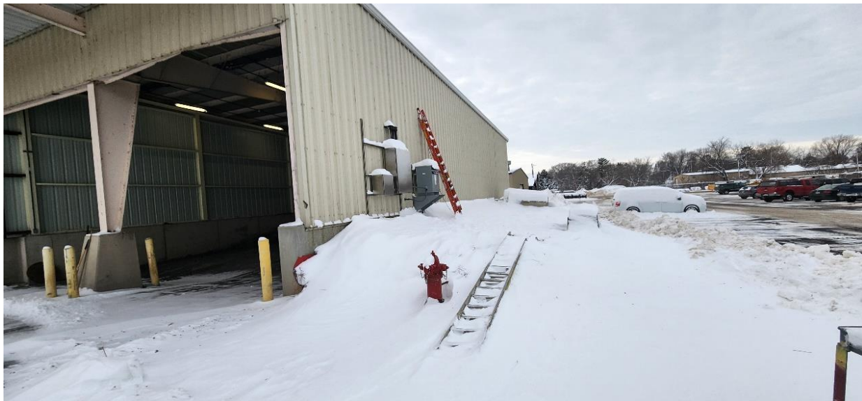
Power and controls moved to exterior of building at Structure 760 (Biosolids Storage Building).
