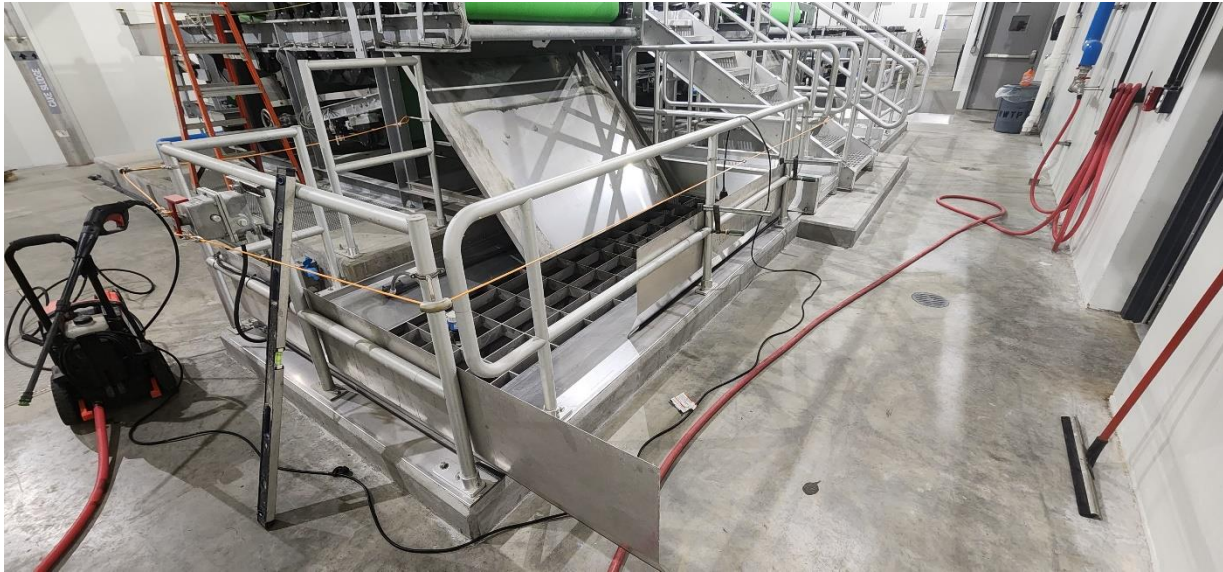
Belt filter press safety plates and hopper collection shields getting installed at Structure 770 (Solids Building).
