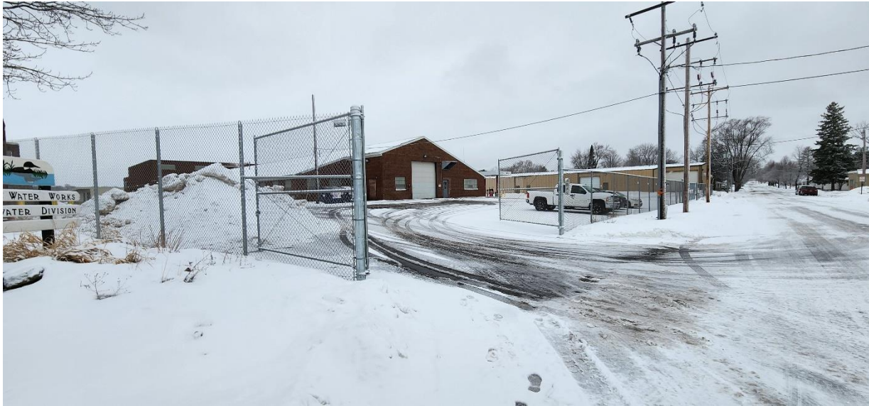
Department of Public Works/WWTF alleyway gate installed for access to Adrian Street.
