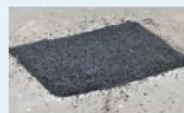
Temporary asphalt repair patch in street and/or sidewalk after service line replacement.
