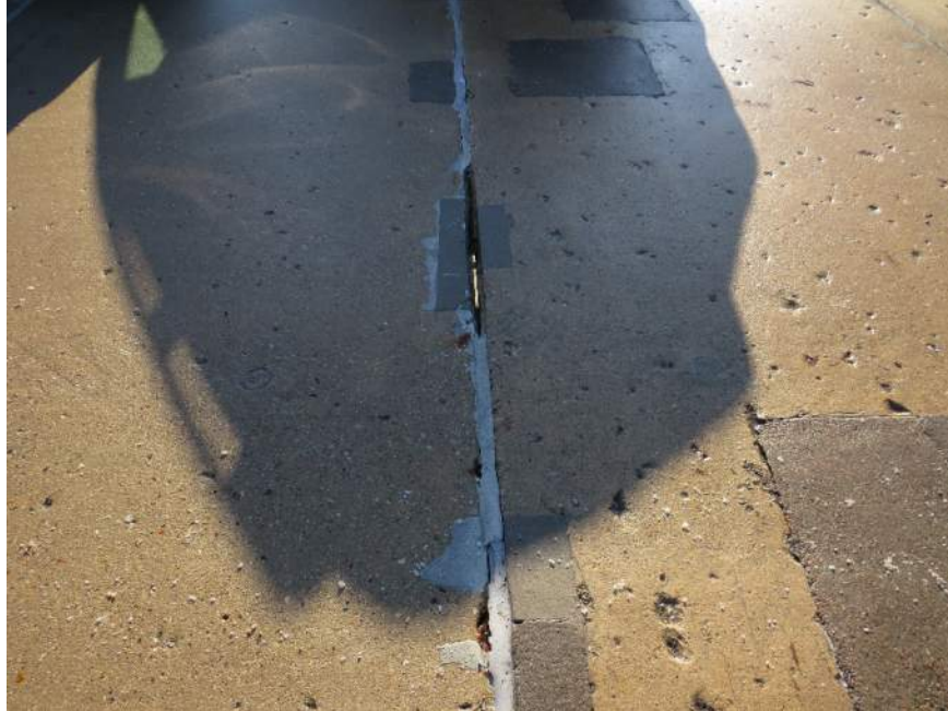
Photo 7. Section of sealant missing, and adhesive failure at double tee joint. Source and Annotation: Walker Consultants (Photo taken 12/8/2022).
