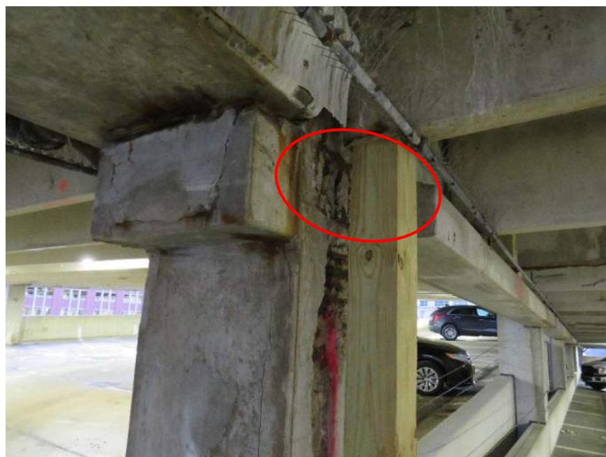
Photo 6. Failed/missing concrete haunch. Double tee is supported by timber post. Source and Annotation: Walker Consultants (Photo taken 12/8/2022).
