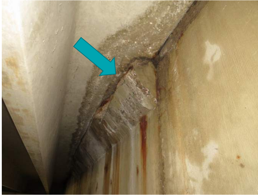
Photo 3. Spall at concrete haunch. Source and Annotation: Walker Consultants (Photo taken 12/8/2022).
