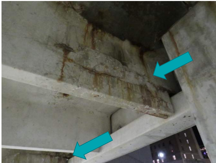
Photo 4. Advanced deterioration at double tee stem. Source and Annotation: Walker Consultants (Photo taken 12/8/2022).
