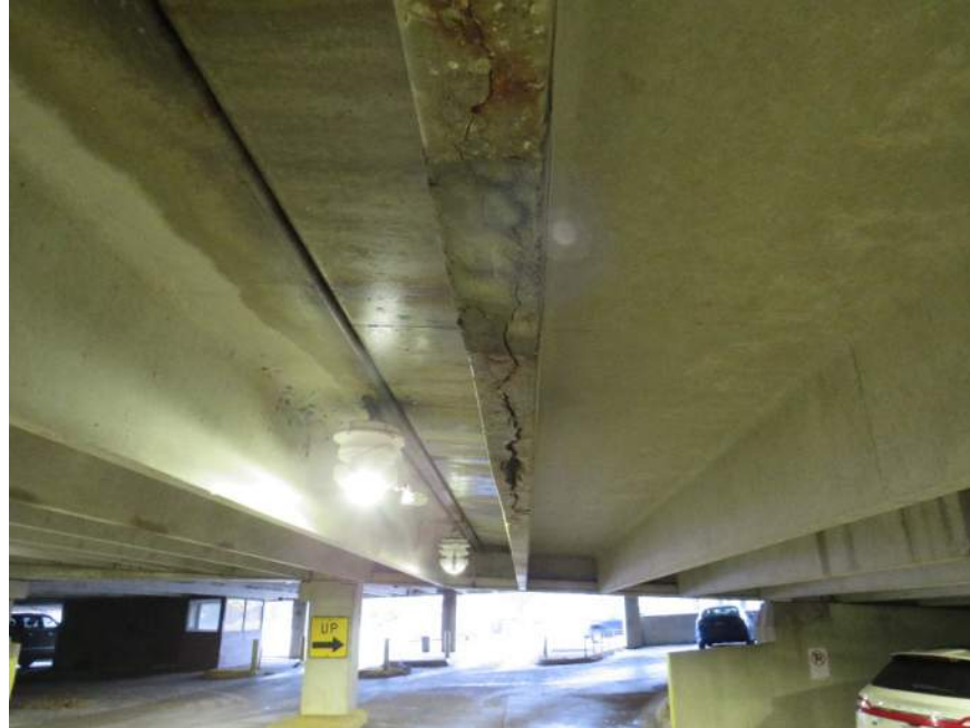
Photo 5. Cracking down the center of double tee stem. Source and Annotation: Walker Consultants (Photo taken 12/8/2022).
